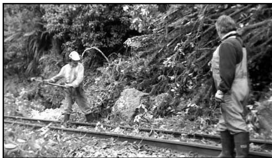
Westport track gangs don't need modern equipment to clear rock from a slip, a sledge hammer is just fine. It's not the norm, however, a slip in the Gorge meant they needed to break a large rock so the LRV could pass.
